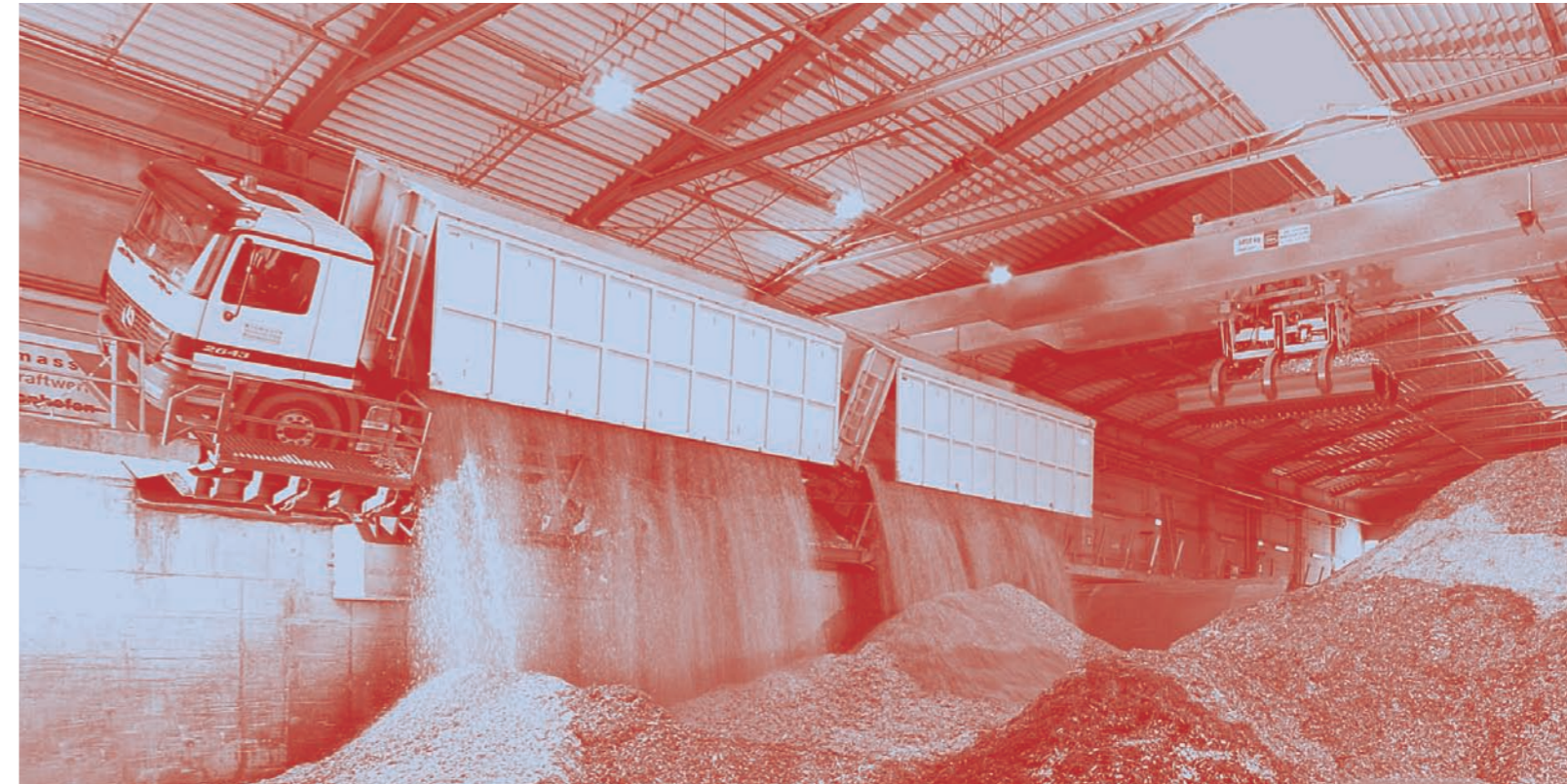
Automatic crane for organic substances heating and power station Pfaffenhofen
